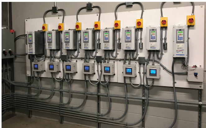
Top: Eco-Flow units with accompanying bypass and Aquatic Controllers. Bottom: A series of Eco-Flow units with Aquatic Controllers.
